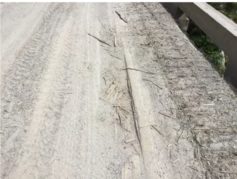
Poor plank condition throughout
