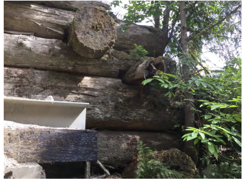
Right bank fill retention tieback log condition
